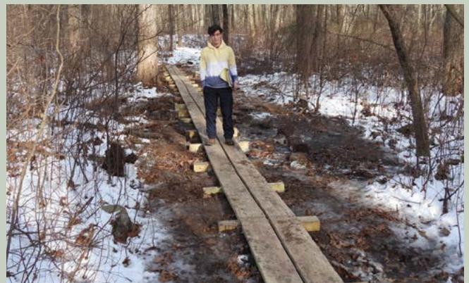
Miles Fraser, Troop 79, constructed an 88 ft. boardwalk on the Nat Smith Reservation for his Eagle Scout Project as the winter became harsh and he had to work around several storms. Photo by Buzz Stapczynski.
